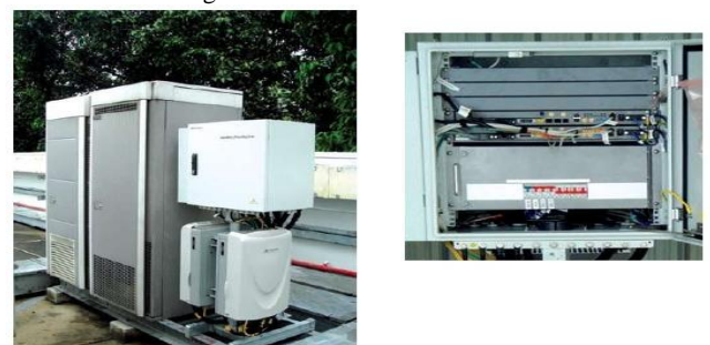
Figure 3 Huawei BTS 3036A [7]
